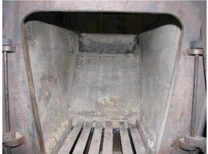
Final result. High temperature cement is used to hold the bricks together and seal the leaks.
